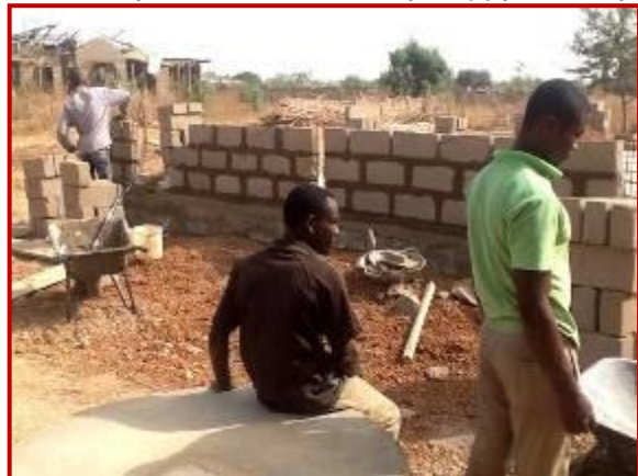
Construction work is in progress on our new Science Laboratory. The work is at foundation level.
